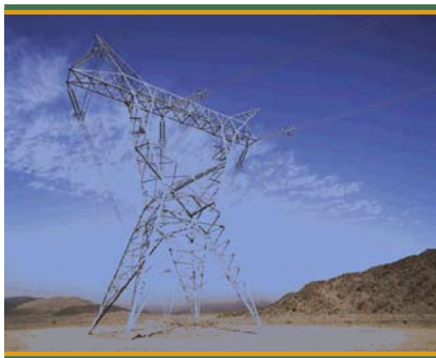
Fig. 7: Transmission Pole: Namibia
