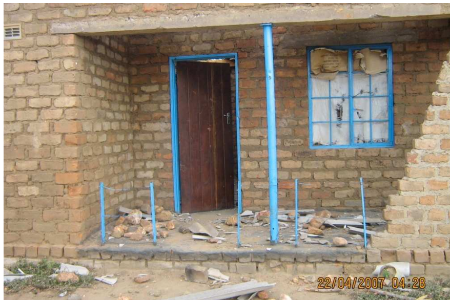
Levy's main house was extensively damaged in a suspected petrol-bomb attack (see more pictures below)
