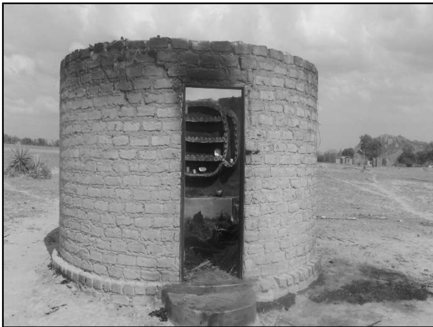
This is what remains of David Chamanga's house burnt in suspected politically motivated violence in Mutoko East.
