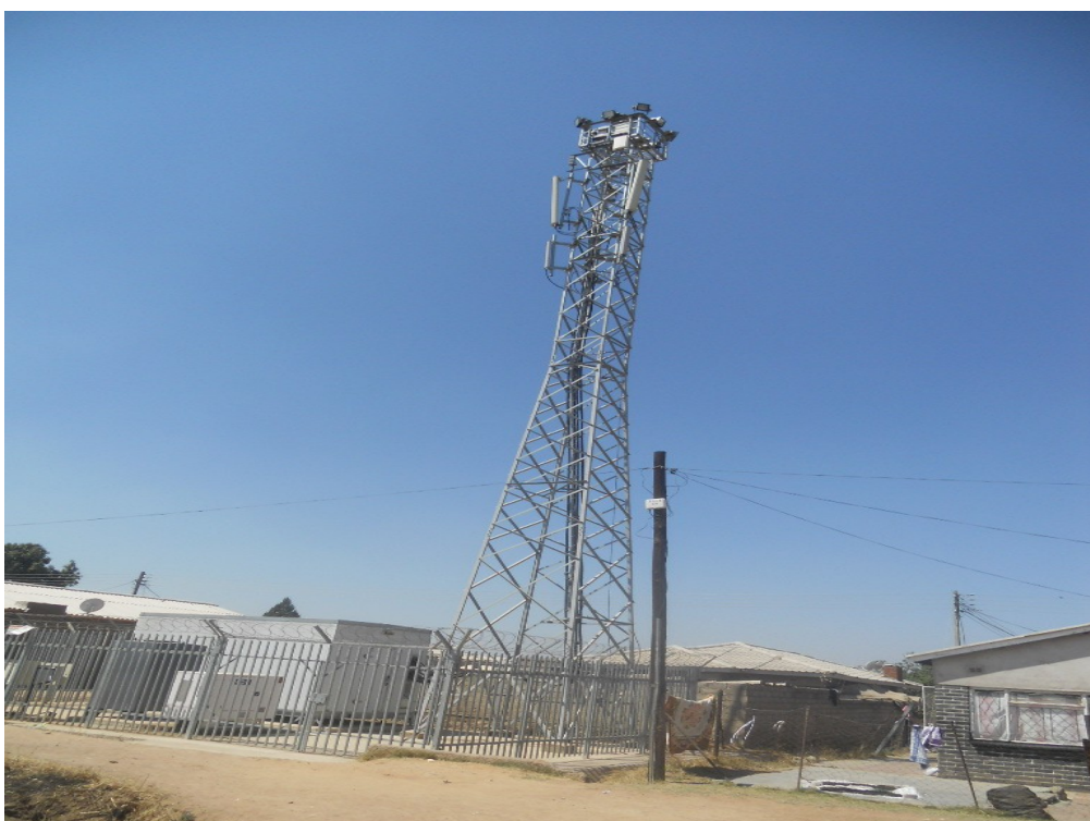
Tower light converted in to a base station.
