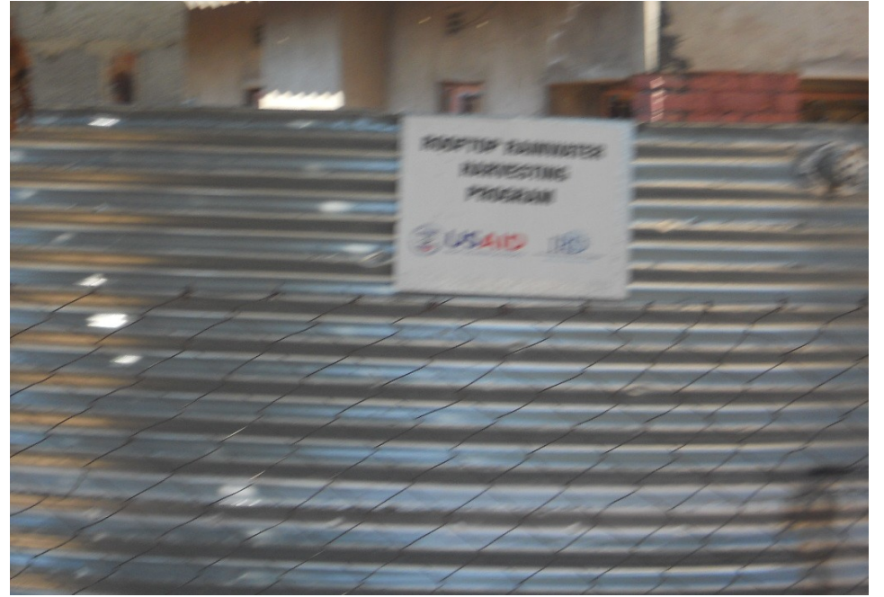
USAID sponsored rooftop water harvesting tank in Unit O.
